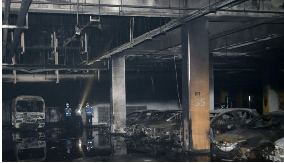
(a) Underground parking fire (Songdo, 2016)
