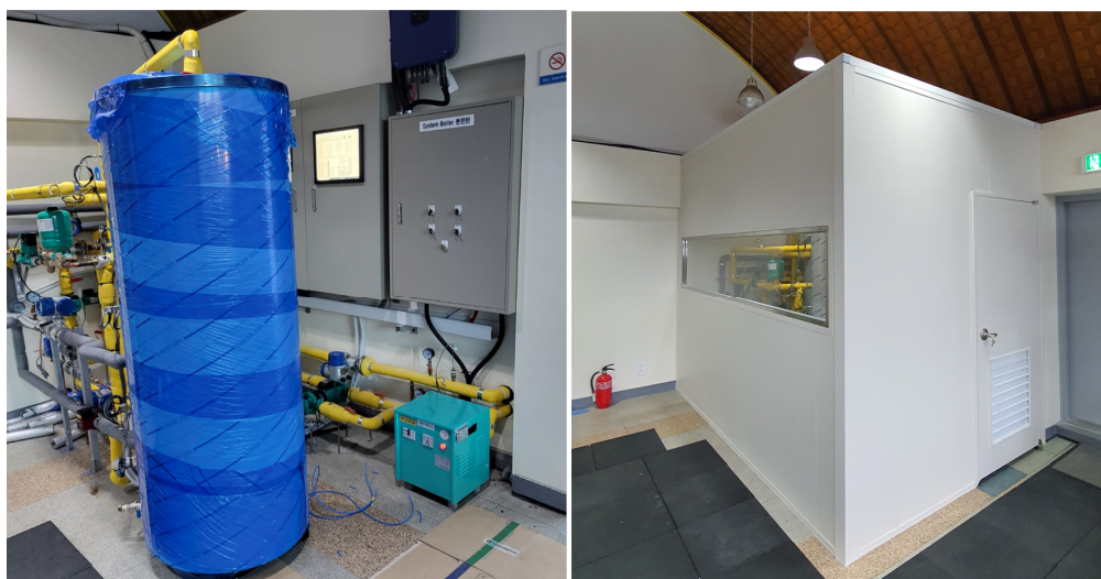
Fig. 7 Machine room view that demonstration system is installed
